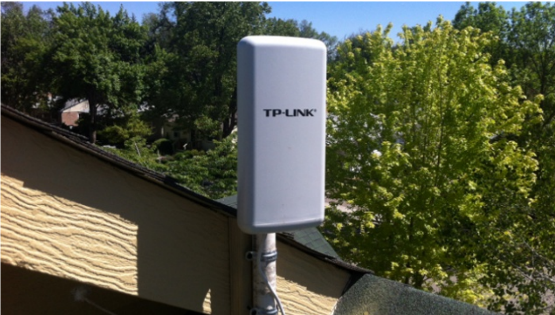
Access point WiFi
