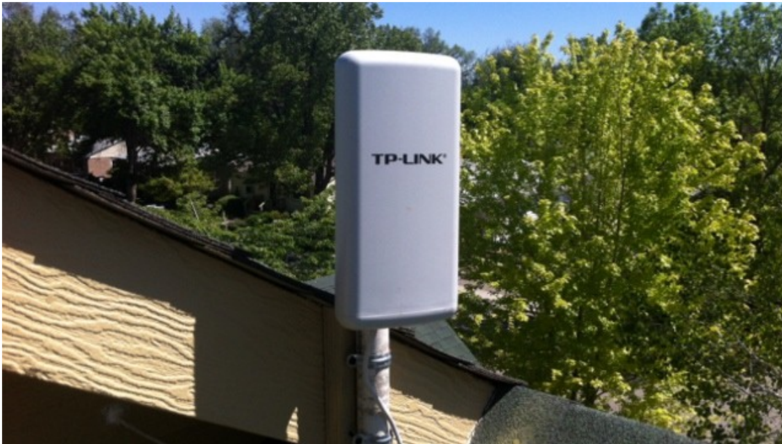
Access point WiFi
